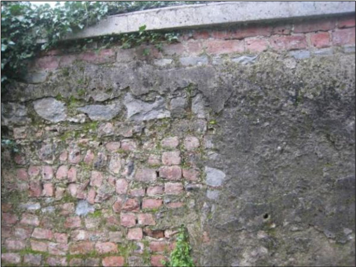
Photograph 56 Section of remaining pre-1840 boundary of the walled garden of Summerville House
